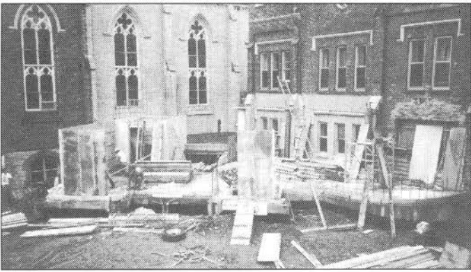
The main floor is in, the foundation has been back-filled, and the main floor walls started. The new elevator can be seen to the back left.
